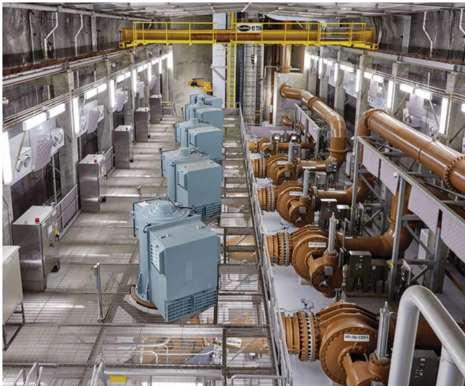
A look inside the ETDPS cavern that pumps 160 mgd to dewater two CSO storage tunnels and convey flow to the Easterly Wastewater Treatment Plant within a 24-hour time frame.
